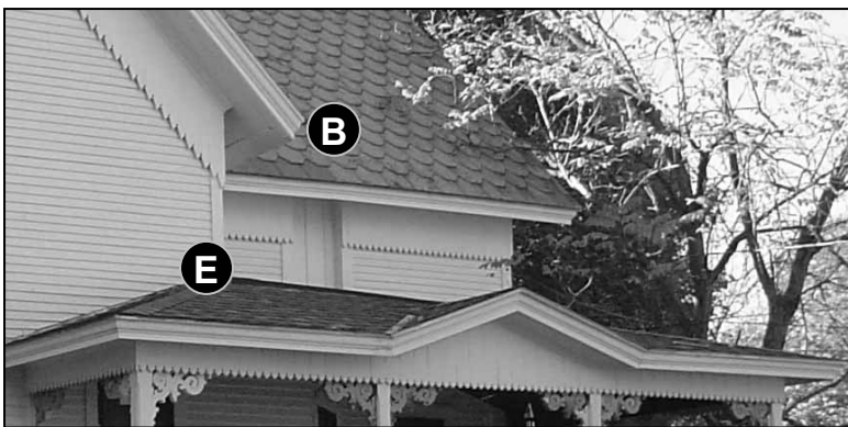
Fig. 5-39: 125 Jefferson St. New slate has been used here to replace portions of the roof that have been damaged.
