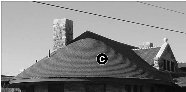
Fig. 5-37: 150 Depot St. The sweeping curve of this roof defines much of the character of the building, and should not be changed or added to.
