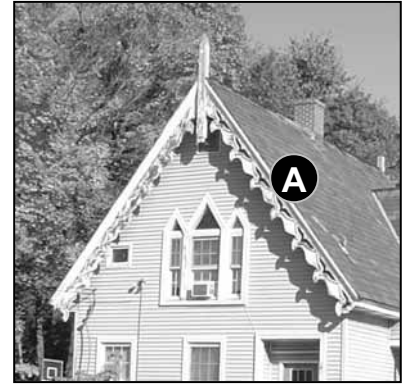
Fig. 5-36: 207 Depot St. The intricate trim details of this eave define much of the character of the entire home, and should be preserved whenever possible.
