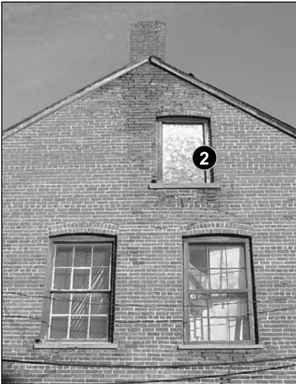
Fig. 5-28: 512 Main St. Windows that are no longer used should not be boarded up or filled in on the outside. Instead, the wall can be in-filled on the inside, leaving the existing window to remain on the outside.
