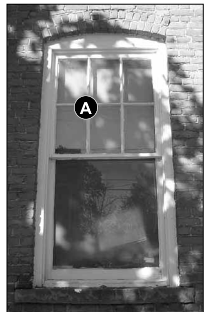
Fig. 5-17: 120 Benmont Ave. It is best to try to repair existing historic windows before replacing them altogether.
