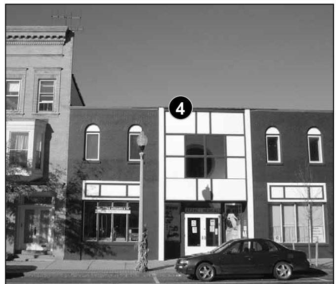
Fig. 5-29: 532 Main St. The original building façade here has been replaced with a large, post-modern window in the center which is inconsistent with the building and its surroundings.
