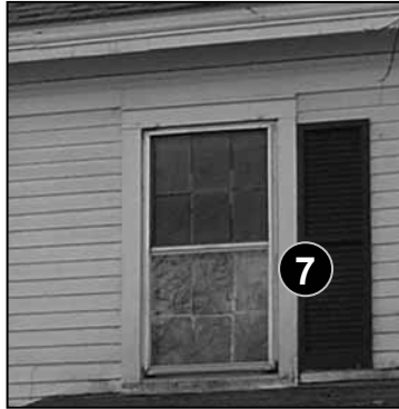
Fig. 5-22: 105 Holden St. Window shutters should be used realistically and consistently on a façade. The imitation window shutters like the one shown here are often seen used on only one side of a window, or on alternate sides of a pair of windows. Such installations are not historically accurate.
