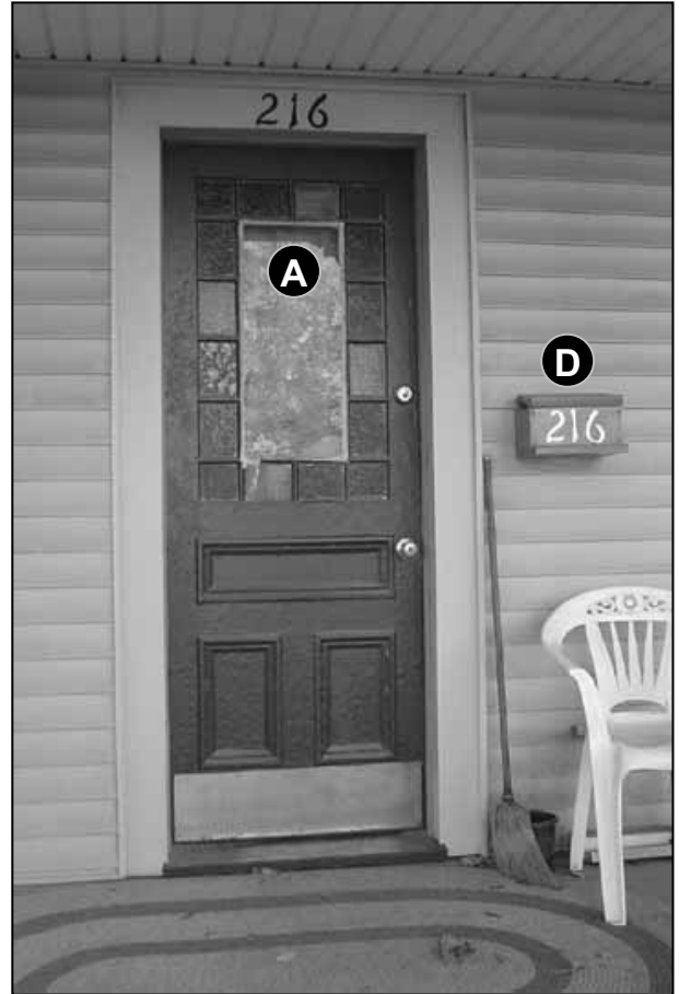
Fig. 5-15: 216 Park Street. The existing colored glass doorway on this house has been preserved and left visible, however the metal kick-plate on the bottom could be painted to match the door to make it less obvious.
