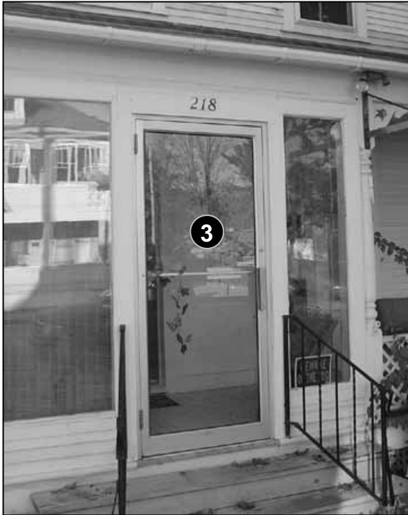
Fig. 5-12: 218 Park St. The commercial storefront door shown here is not appropriate on a residential structure.
