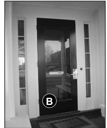
Fig. 5-9: 507 Main St. The storm door which has been added here is designed to match and reveal the original front door behind it.
