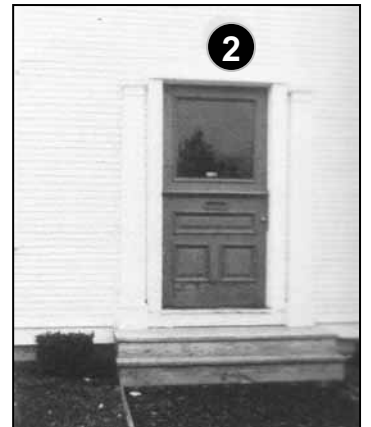
Fig. 5-11: This entryway has been altered by the removal of the original woodwork found above the door. [Date unknown.]
