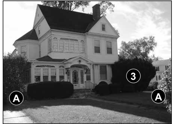
Fig. 5-56: 217 Main St. The large bush to the right of this house has overgrown and may cause moisture damage to the exterior.
