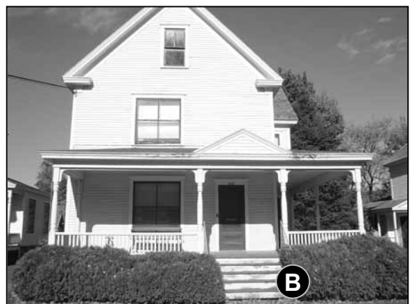
Fig. 5-60: 204 Main St. These hedges have been trimmed to keep from overwhelming the porch, but could be trimmed more in the back to prevent water damage to the porch.
