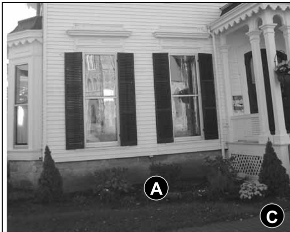
Fig. 5-57: 213 Main St. Small shrubs along the foundation of the building still allow sunlight, ventilation and access for maintenance.
