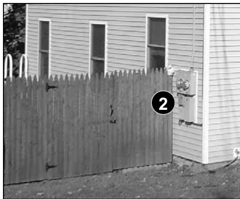
Fig. 5-63: Corner of Weeks & Jefferson. Although the electric meter has to be accessible, it doesn't need to be so visible.
