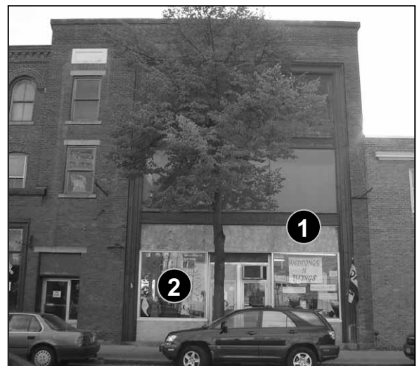
Fig. 5-84: 337 Main St. Original storefront has been replaced with bare aluminum framed picture windows and blank, unfinished panels.
