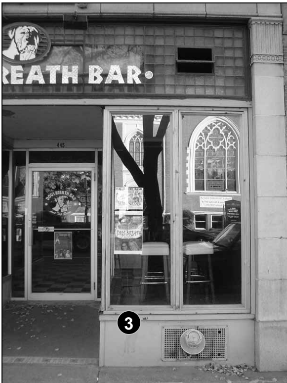
Fig. 5-83: 449 Main St. Bare lumber framing for the storefront windows is not in keeping with historic designs.
