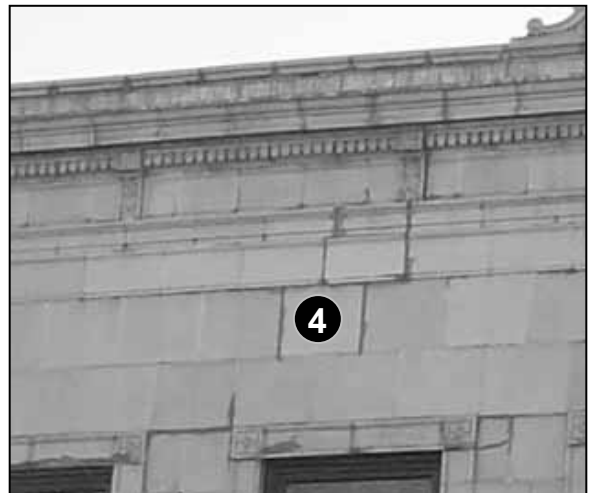
Fig. 5-35: 449 Main St. Joint repair which uses the wrong mix or mortar can result in highly visible joints. Be sure that test-mixes are tried before real work commences.
