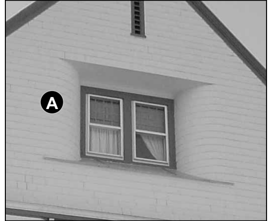
Fig. 5-30: 124 Elm St. Original curved shingles are used here to highlight the sculptural nature of the façade enclosure.
