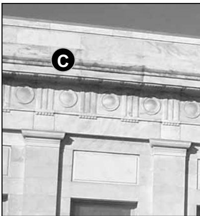
Fig. 5-32: 118 South St. Light colored stone surfaces such as this often need to be cleaned, but the cleaning process should never permanently change the appearance of the materials.
