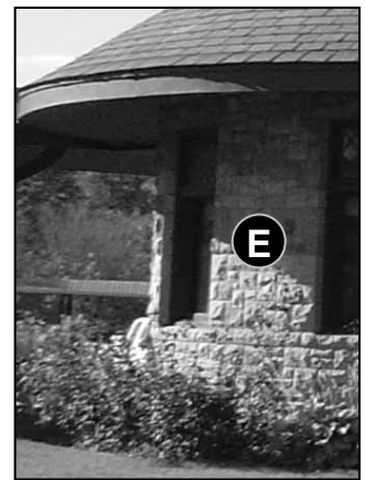
Fig. 5-34: 150 Depot St. This rough ashlar masonry wall surface adds texture and depth to the façade.
